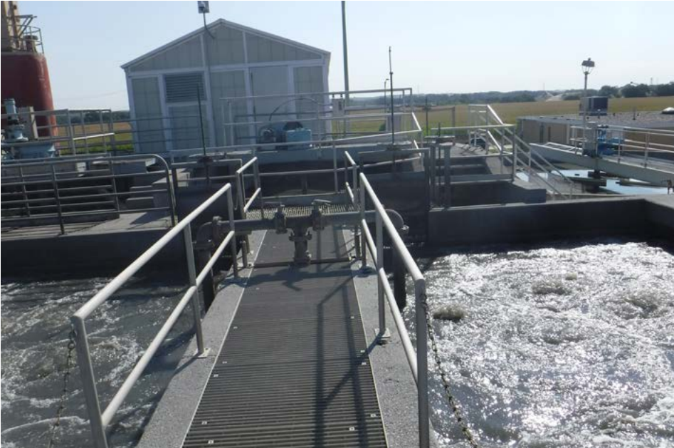
The current Water Pollution Control (WPC) grit removal system is 50 years old and has limited capacity.
